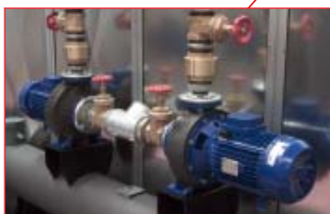
Pump and stand by pump reserves with interception valves Pumpe und Stand-by-Pumpe mit Absperrventilen
